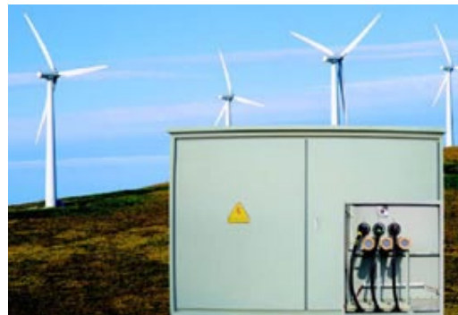
35kV plug-in termination in cable branch box
