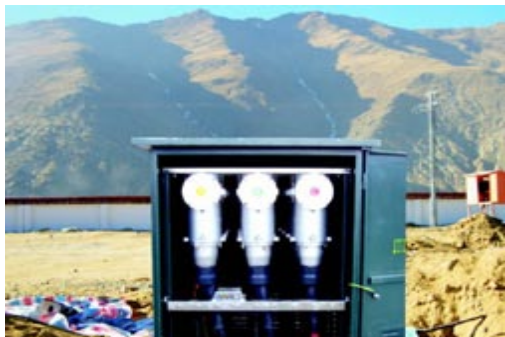
35kV plug-in termination in cable branch box installed in Tibet railway
